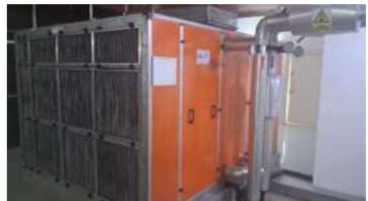
Typical AHU (part of Subject Property) on all floors of Subject Tower
