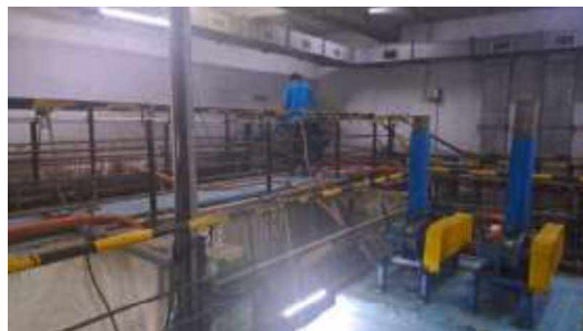
Internal View of STP in Subject Tower
