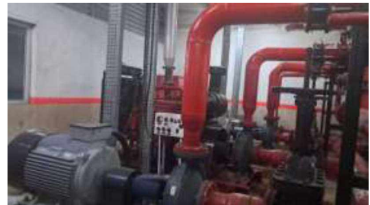
Internal View of Pump Room in Subject Tower
