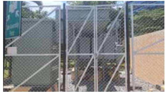
View of electric substation at ground level of Subject Project
