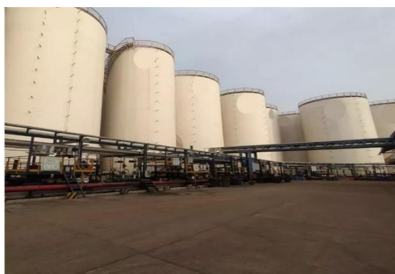
Storage for liquid products Deendayal Port, Kandla
